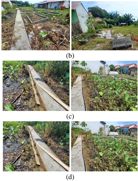
Figure 6. The results of the pathway construction work. (a) results in the first and second days. (b) developments in the third and fourth days. (c) developments in the fifth and sixth days. (d) products on the seventh and eighth days.
