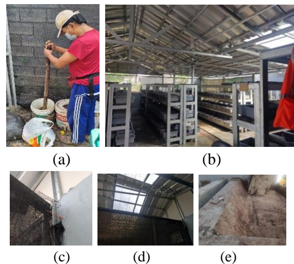
Figure 8. Some of the physical conditions of the maggot house (a). crushed manually, (b). dark maggot house, (c). leaking fly cage, (d). low sunlight, (e). slope biopond
