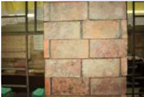
Plate 12. A column done with modern tools and procedures using the same brick as the chief material but mixed with concrete rather than stucco plaster. Resembles a modern decorative stone effect rather than reconstructing the original.
