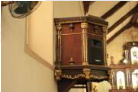
Plate 9. The pulpit panel, historically destroyed by the introduction of an electronic speaker in recent renovation works.
