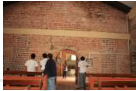
Plate 14. The interior wall of the Adoration chapel. The original location of windows are covered with bricks to recreate the same material but destroyed the uniformity of the brickwork pattern. Also shown is the exposed electrical wire moulding attached to the brick wall.
