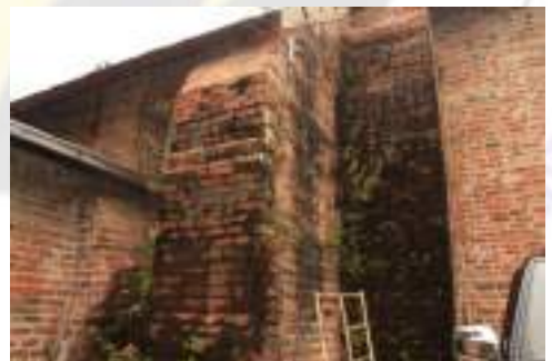
Plate 6. A support buttress covered in algae and moss. Upon closer look, water has already penetrated a portion of the core and slowly washing away the mortar and plaster that bind the bricks together.
