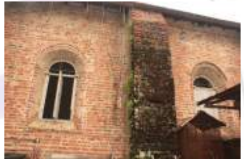
Plate 5. Dilapidated windows and a support buttress invaded by grass, moss and algae.
