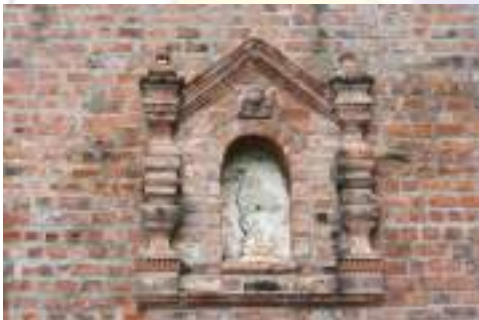
Plate 2. Detail of the belltower façade. The century old original image of the patron saint inside the arch was allegedly stolen.
