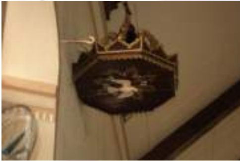
Plate 9. The detail of the pulpit's overhead cover. Paint is obviously peeling off and needs to be restored.
